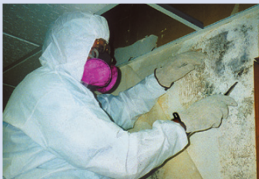
Photo 7: Remediation worker with limited PPE
