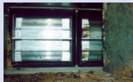
Photo 4C: Moldy air duct
