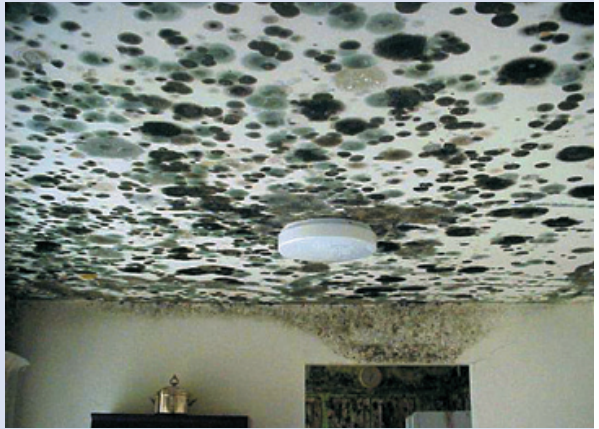
Photo 2: Extensive mold contamination of ceiling and walls
